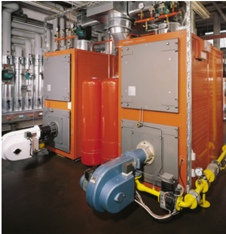
Gas inlet pressure monitoring on high-performance boilers
