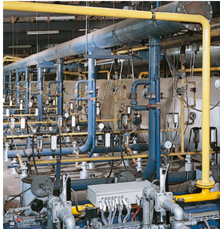
Gas train in a brickworks
