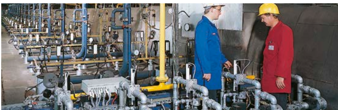
Gas train in a brickworks
