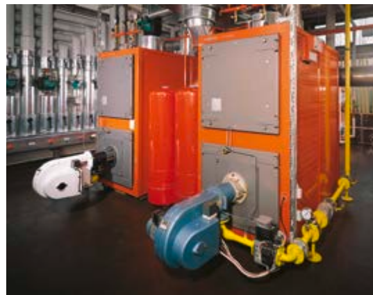
Gas inlet pressure monitoring on high-performance boilers
