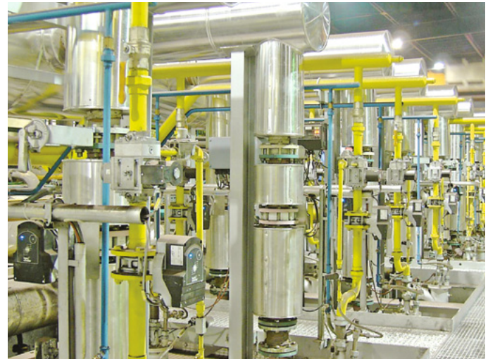
Walking beam furnace with overhead firing
